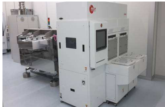
RECIF 450mm EFEM installed in imec clean room
